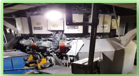
Packing Plant Conweigh 3No x 180 TPH, Fls : 1No x 120 TPH
